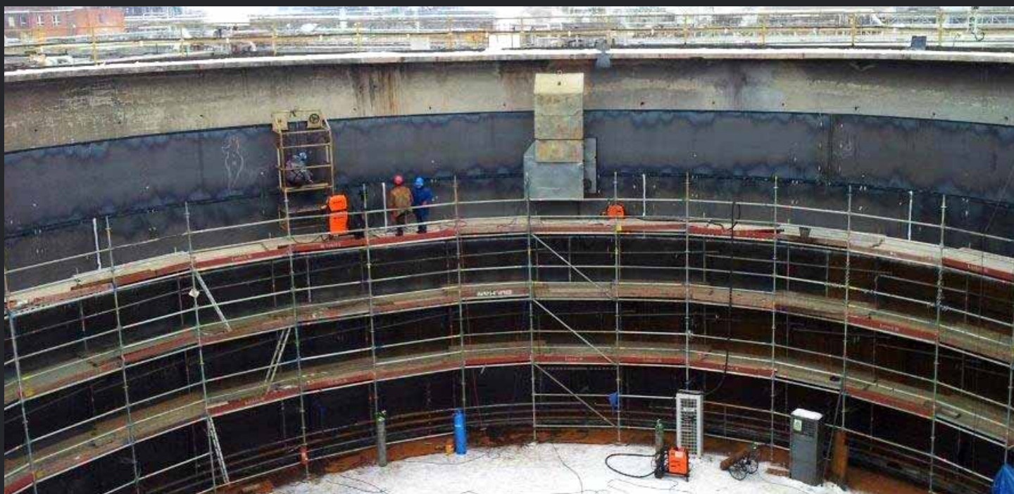
Euromont Group a.s., construction of a new tank in Kralupy nad Vltavou.
