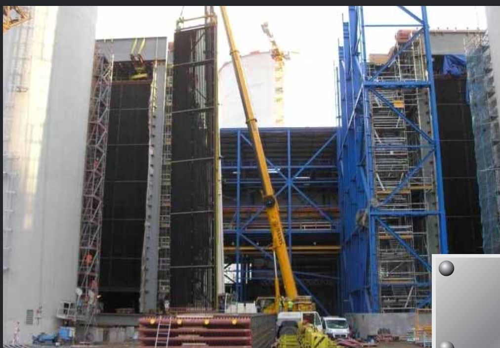
Supply and installation of a steel structure for waste heat boilers K1 and K2 as part of the construction of a new Počerady power plant boiler delivered by PSG - International a.s.
