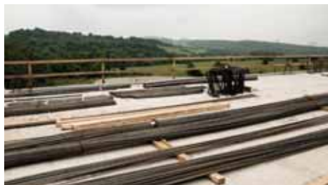
D8 highway, construction No. 0805 Lovosice - Řehlovice, part A – highway line A 215 – highway bridge over road No. III/258 29 ŽIM - Řehlovice
